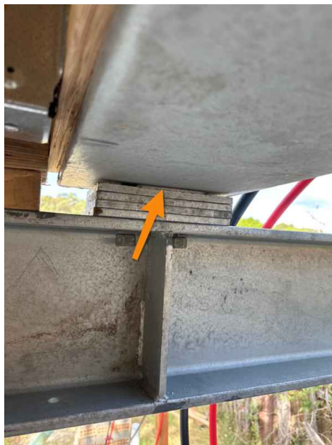
Beam should have 200mm of bearing. Currently the last packer is only 100mm wide. This connection is not as it specified by the engineers drawings
