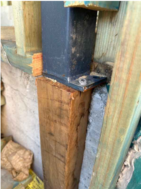
Structural load not designed to bear on timber, this has been done as it appears the slab edge was poured short
