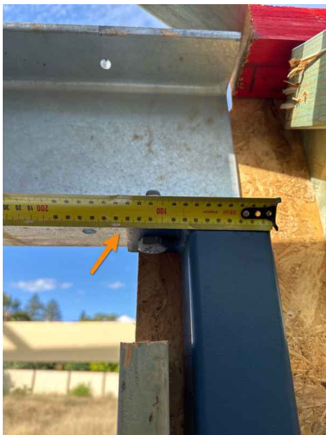
Post plate has been cut short and now only allows a single bolt
